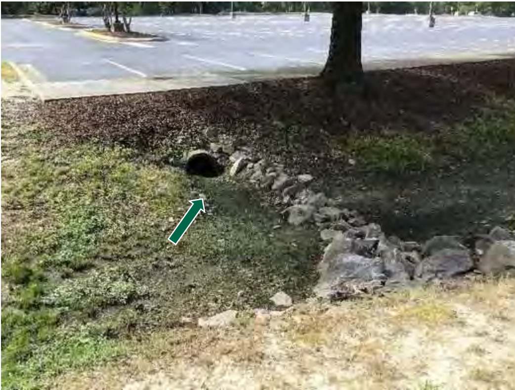
Main Inlet (note accumulated sediment, arrow)
