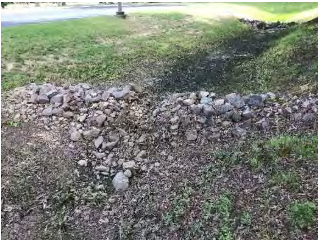
Forebay Checkdam - Appears Clogged with Sediment and Debris (per plans, it should be 3' high on ends and 2.5' high in center)
