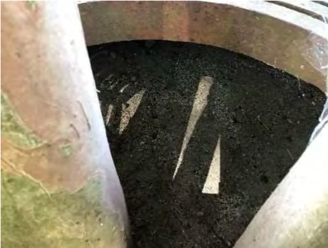
Note Accumulated Road Grit Within Unit
