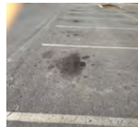
Leaks from vehicles
