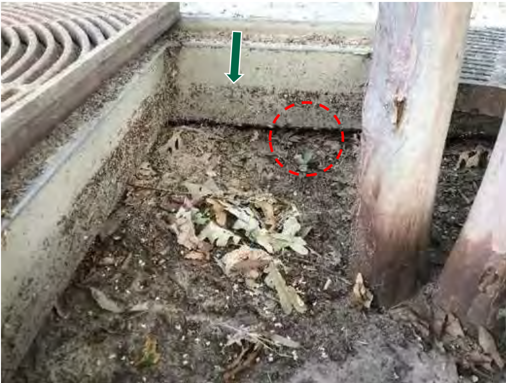
Note High Water Mark (arrow) and Lack of Freeboard Between Accumulated Sediment and Unit (circled)
