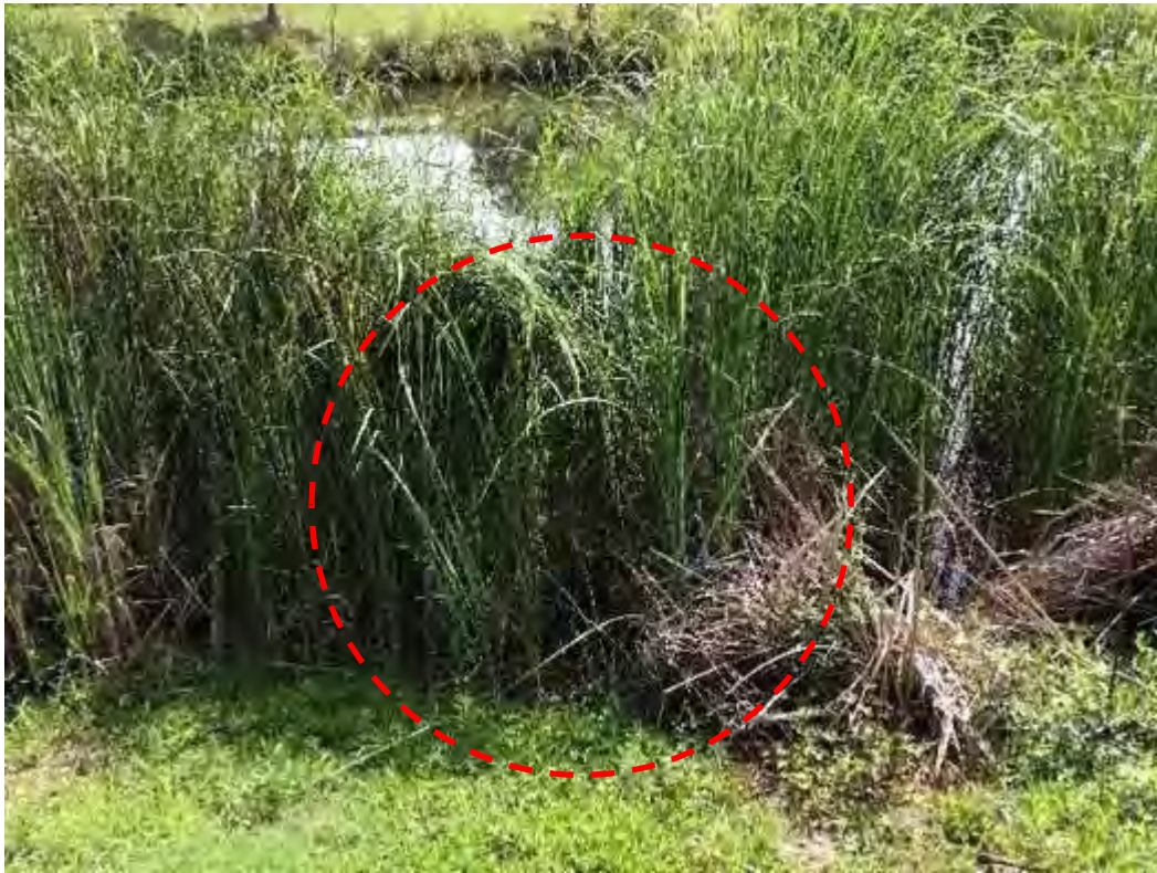
Control Structure (obstructed by overgrown vegetation)
