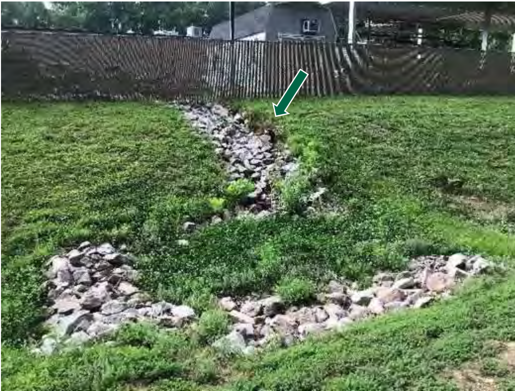
Rip-rap Inlet from Facilities Maintenance Building Yard (note erosion, arrow)
