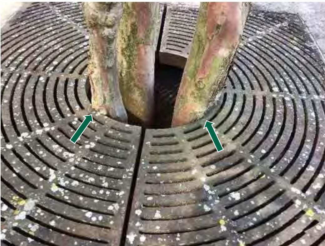
Maintenance Access Grate Cannot be Opened Due to Overgrown Tree
