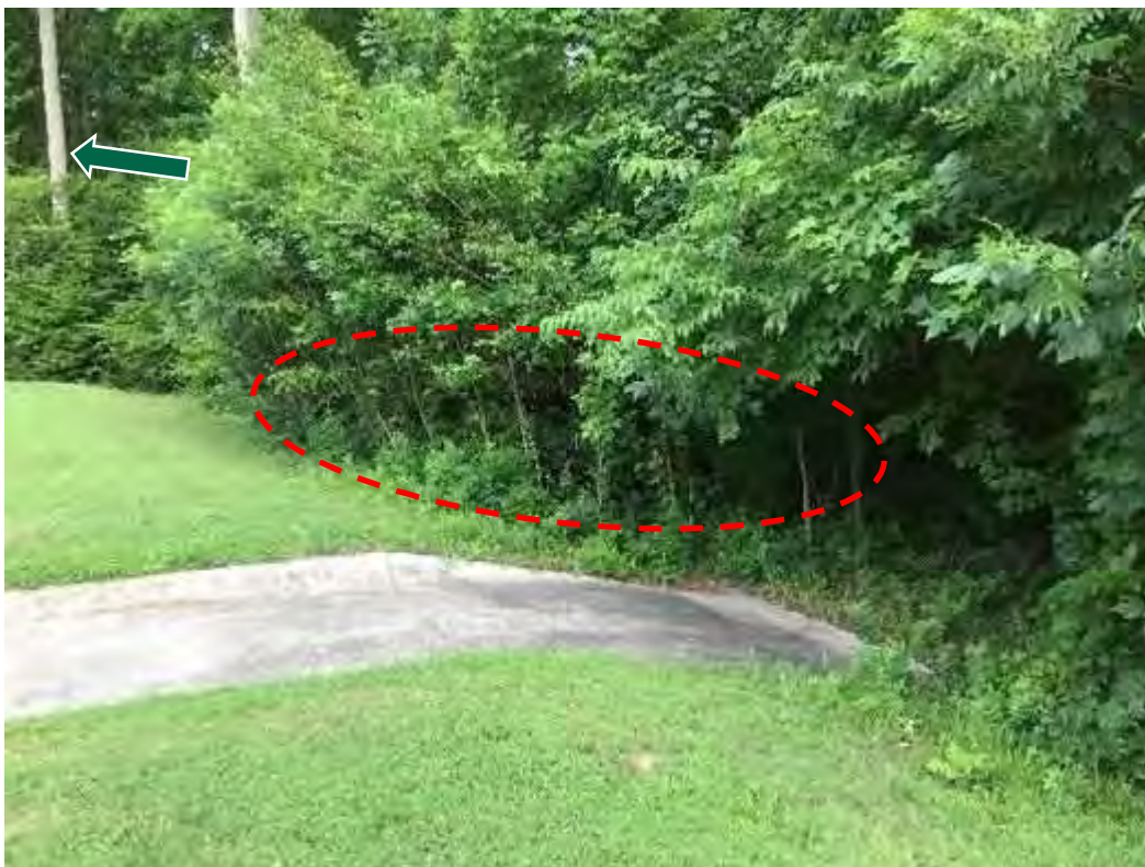
Emergency Spillway and Embankment Downstream Toe Note old trees (arrow) and new trees (circle)
