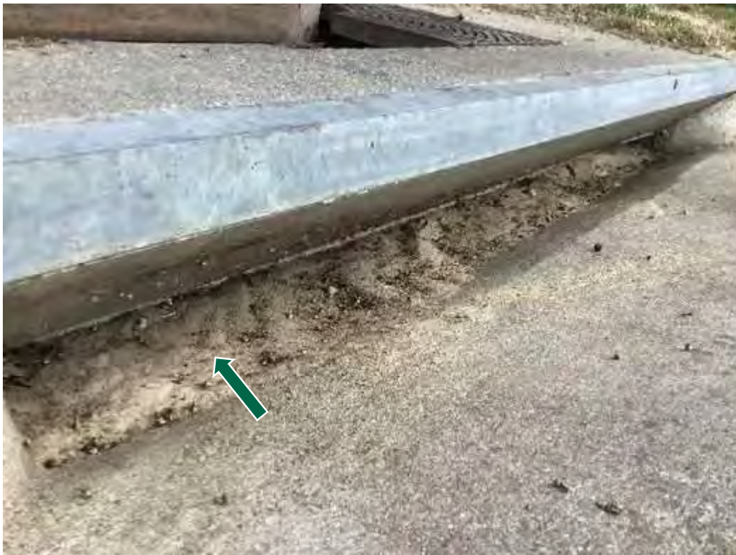
Note Accumulated Sediment and Fines in Inlet Throat
